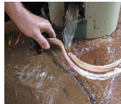
Above: Calcite scale build-up on an electric hot water system element.
