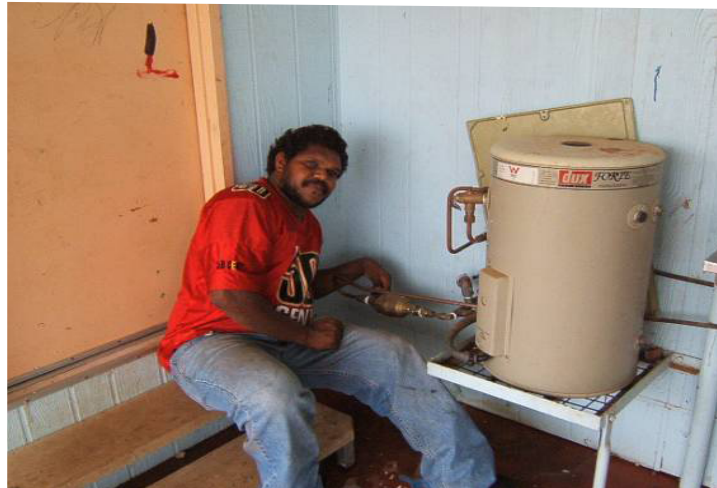
Above: Community ESO Norman Hagan reads a flow meter on a hot water system.
