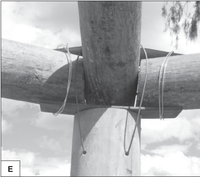
The poles can then be wired together using a Cobb & Co. hitch (photo E).
