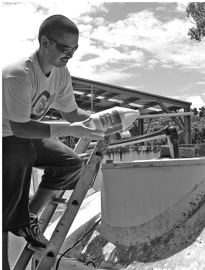
After measuring the volume of water in this tank, Seth added 1 litre of bleach.
