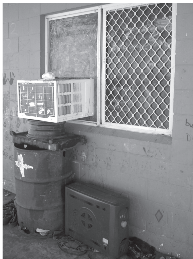
Fig. 1: An air conditioner unit installed by a tenant, and is supported precariously by found objects.
