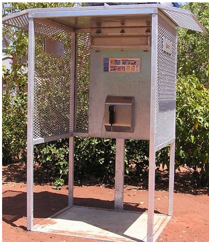
Figure 4: Cabinet mounted Trillium phone on the Dampier Peninsula
