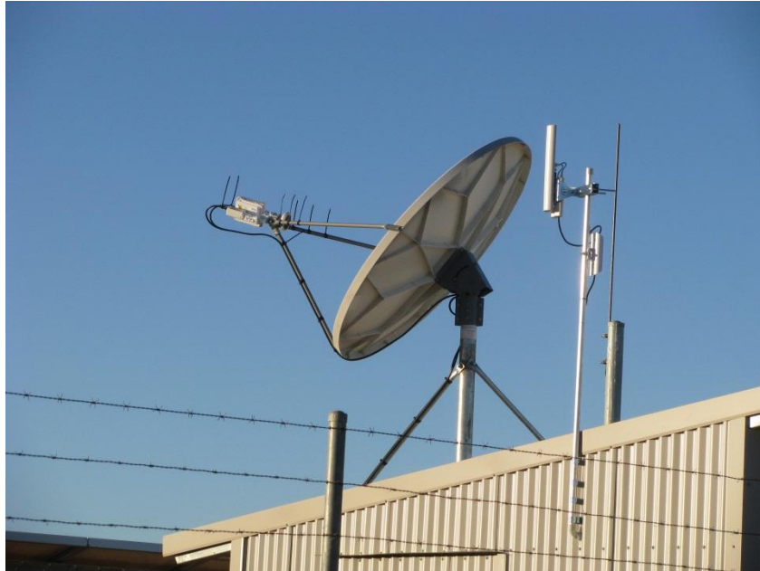
Figure 3 – Part of Mungalawurru Bushlight shelter showing satellite antenna, with central WiFi antennas in the foreground
