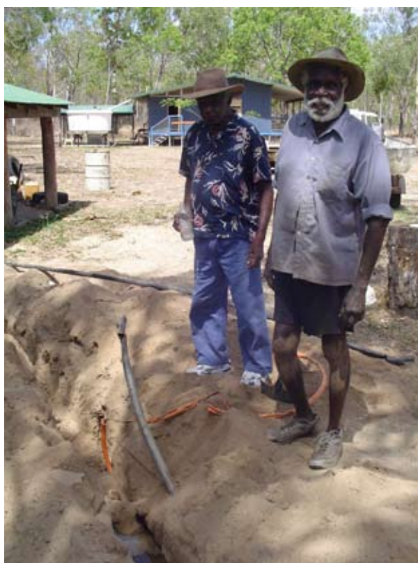
Photo 1: (From left) Sunlight Bassani and Keith Liddy fix the broken water pipeline at Top Camp.
