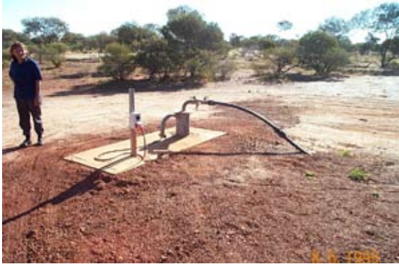
Photo 2: Kanpa residents concreted around the borehead and covered the cables before the skills program started.
