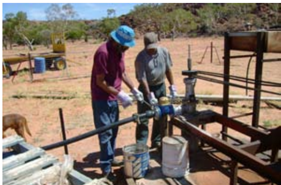
Photo 1: Reg and Peter Kenny install a water meter at the Mpwelarre borehead.
