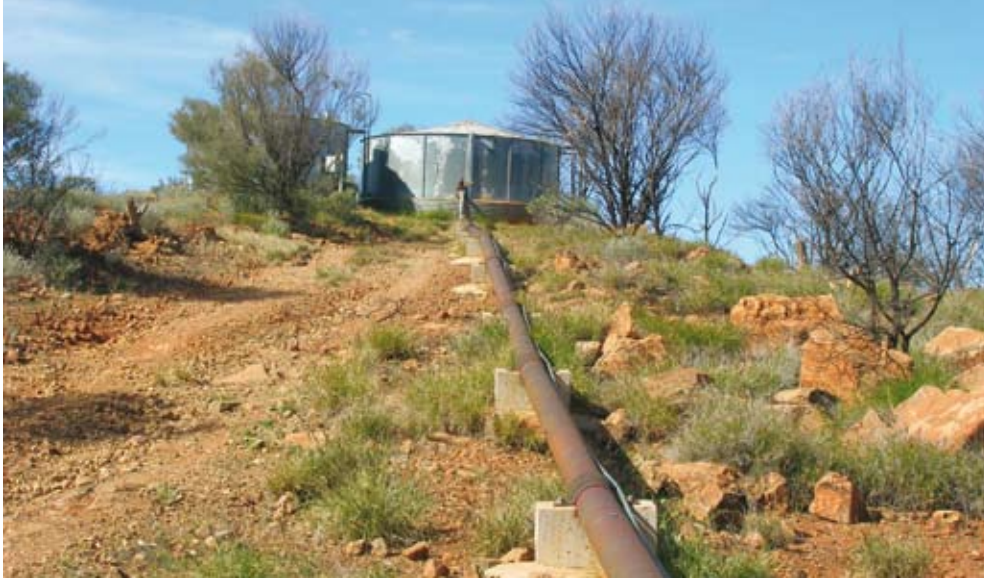
Figure 24: Water storage tanks
