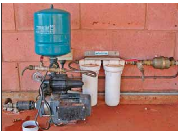
Figure 9: The pump and water treatment system installed in the case study trials. The filters are encased in the white cartridge holders.
