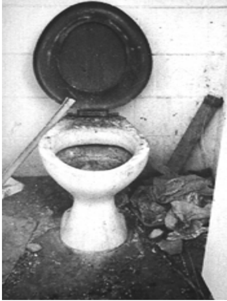
Figure 13: Dual Flush Toilet that was installed into a remote Indigenous Community
