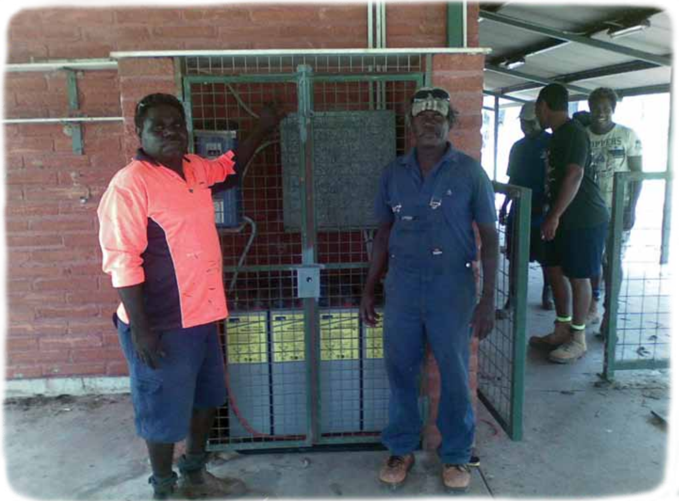
Maningrida course participants in front of battery storage tank.
