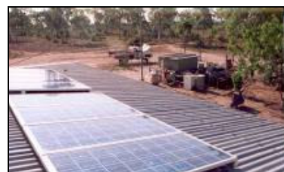
Solar Panels on house
